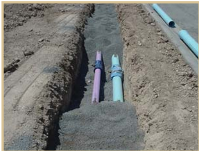
Dual reticulation at Pimpama Coomera. Using recycled water as an alternative water source was a major part of the master plan.
