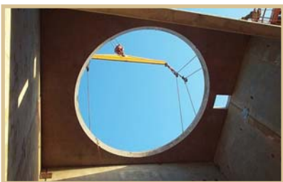
Every part of this construction was precast elsewhere in Australia and transported to the site.
