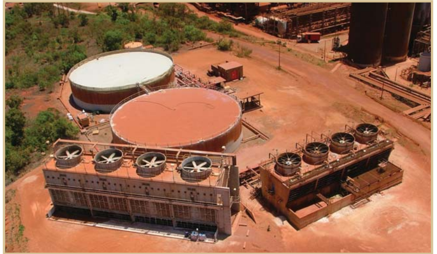
Aerial view of the Gove water cooling tower, three years after completion (Photo: ALCAN Engineering)
